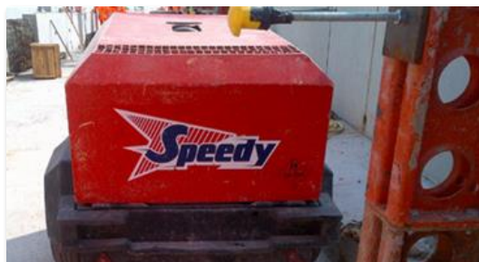
Generator with no drip tray in place
