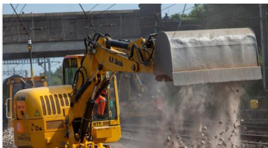
Going to enter a site where ballast dust is being created without proper protection
